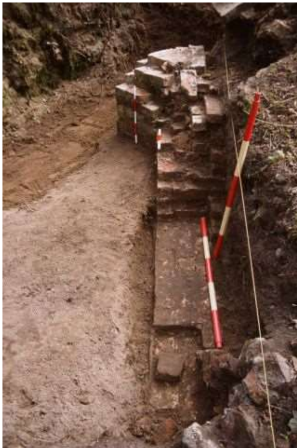
The demolished stretch of Monks' Walk wall and the buttress, looking South towards the Mount
