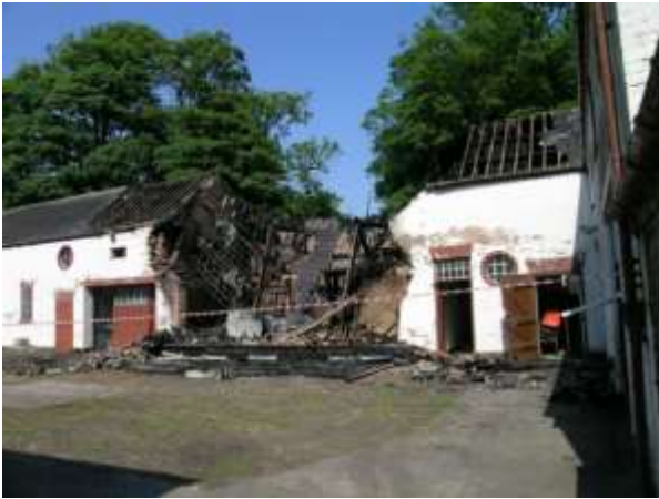
Fire damage at the Stables (East block)
