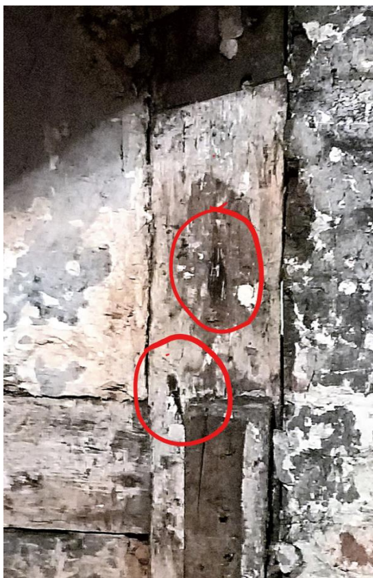
Burn marks found under stairs at Lytham Hall
