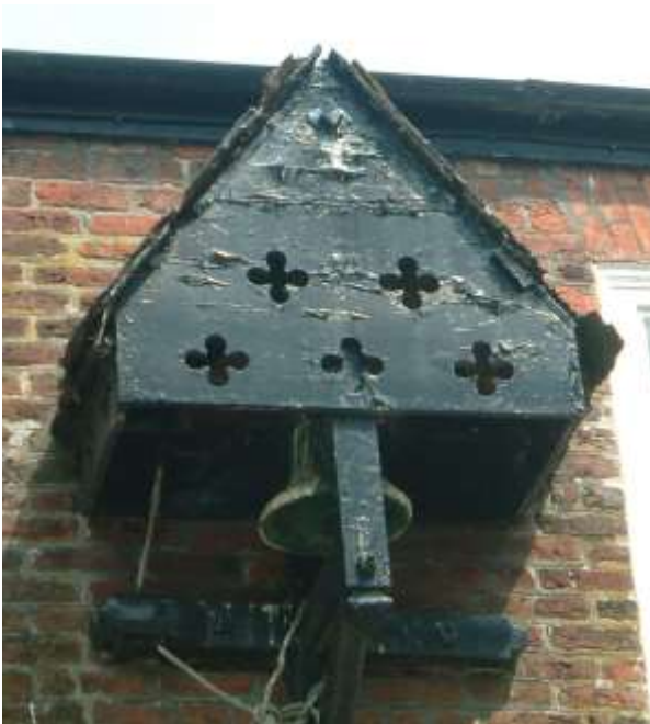
The Rear Courtyard Bell needs attention
